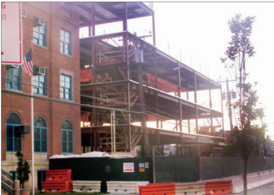
Work at the new PS 256 was halted for 3-4 weeks following a construction mishap.
